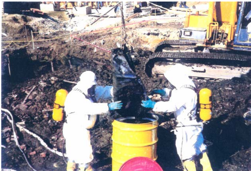
Hazardous Drums Cleanup
